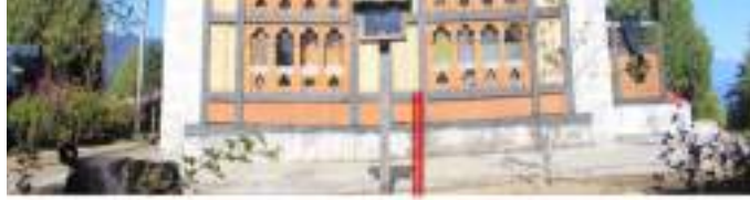
Cracks on the wall and timber components of rabsel due to earthquake.
