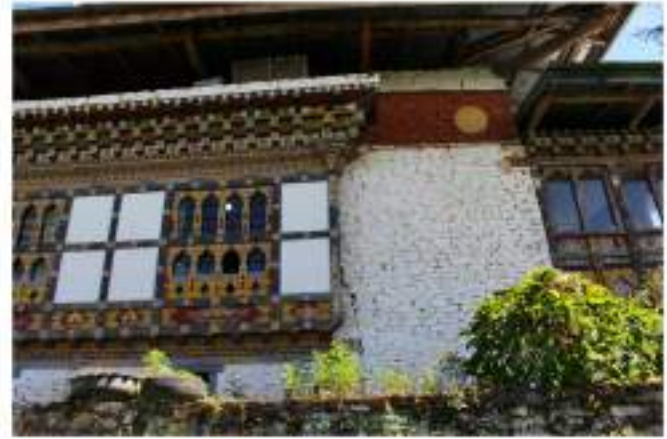
B. Vertical Crack at the connection of rabsel & wall
