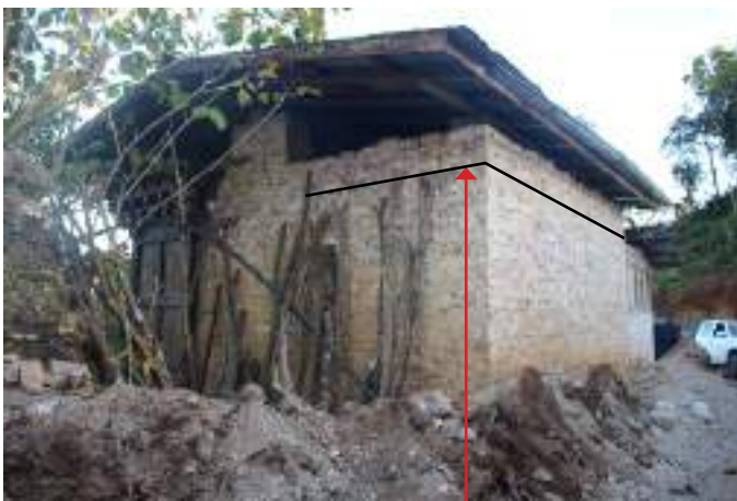
No keymar on the external wall
