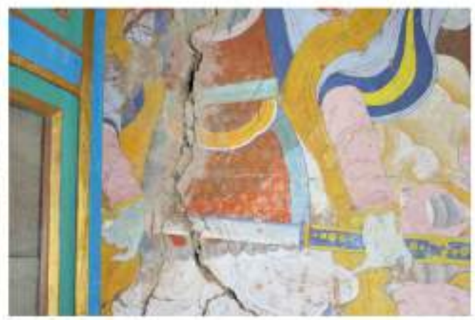
D. Vertical crack in the interior of the lhakhang
