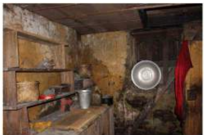
D. Caretakers room walls soaked wet from the water seeping from cliff behind
